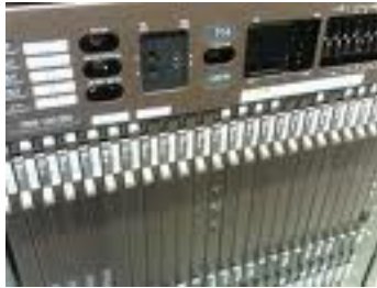
Figure 2: Nortel Networks DMS-100 Central Control
